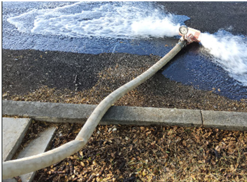
Figure 6-7 Hose with a Pitot Gauge and Diffuser
