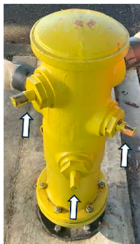
Figure 6-3 Hydrant Stem Nuts
